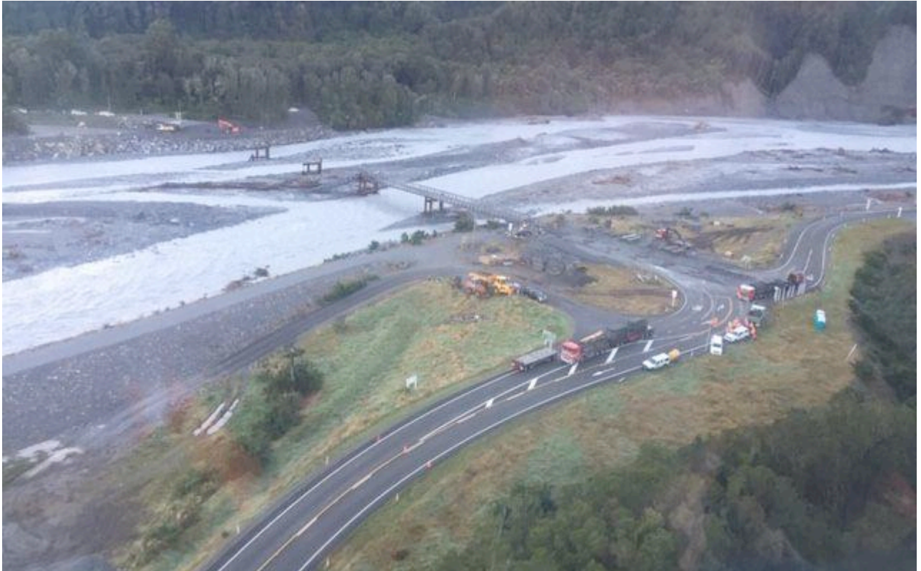
Figure 16. Damaged Waiho River Bailey Bridge after torrential rain in March 2019. Source: RNZ, 2019.
